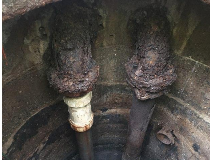
Figure 8. Corroded discharge piping in lift station #18 wet well.
