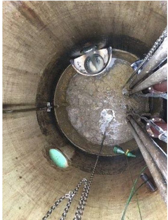
Figure 2. Eardley lift station significant grease mat.
