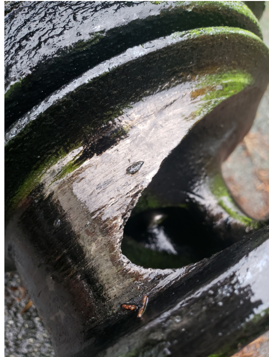
Figure 7. Reduced impeller profile and compromised impeller geometry due to wear in the Beach Comber lift station.
