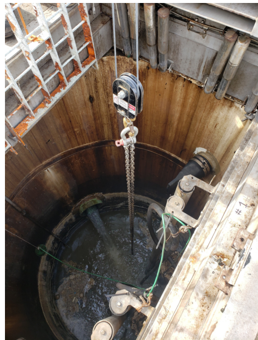
Figure 3. #12 lift station with visible corrosion on fall protection grating.
