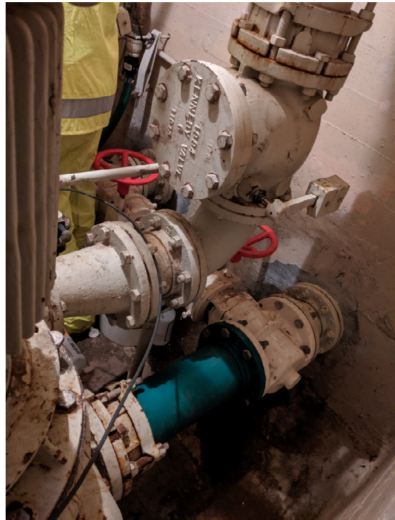
Figure 6. Red-handled isolation valving in the Arena lift station.
